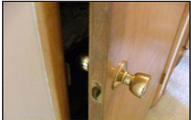
Hall, bathroom doors don't latch; repair.
