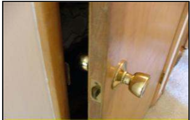
Hall, bathroom doors don't latch; repair.
